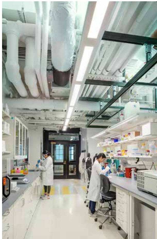
Lab buildings like this one on a Cambridge, Massachusetts, research campus, with their heavy demands on air flow and energy use, play a key role in how campuses are targeting greenhouse gas emission reductions.
